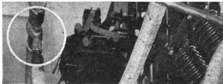
CLOSE-UP VIEW OF WESTINGHOUSE-FRANKEL CABLE TAP (WITH INSULATION REMOVED) IN PLANT OF FLATBUSH GAS COMPANY, BROOKLYN, N. Y.
